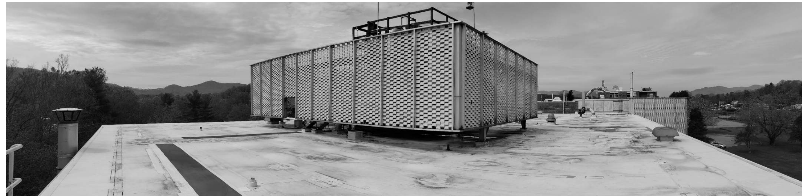
D.5 OVERALL VIEW OF AREA D FROM PLAN EAST. COOLING TOWER AND SCREEN TO BE REMOVED. COORDINATE WITH PME DRAWINGS. EXISTING STEEL EQUIPMENT STANDS TO REMAIN. SEE G6/A402 FOR EQUIPMENT STAND DETAIL
