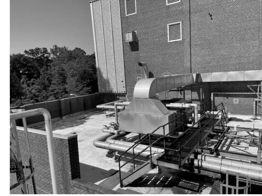
B.15 OVERALL OF SOUTHERN EQUIPMENT AREA. EQUIPMENT TO BE REMOVED. EACH PARAPET CAP CONDITION IN PHOTO IS UNIQUE. SEE DETAILS.
