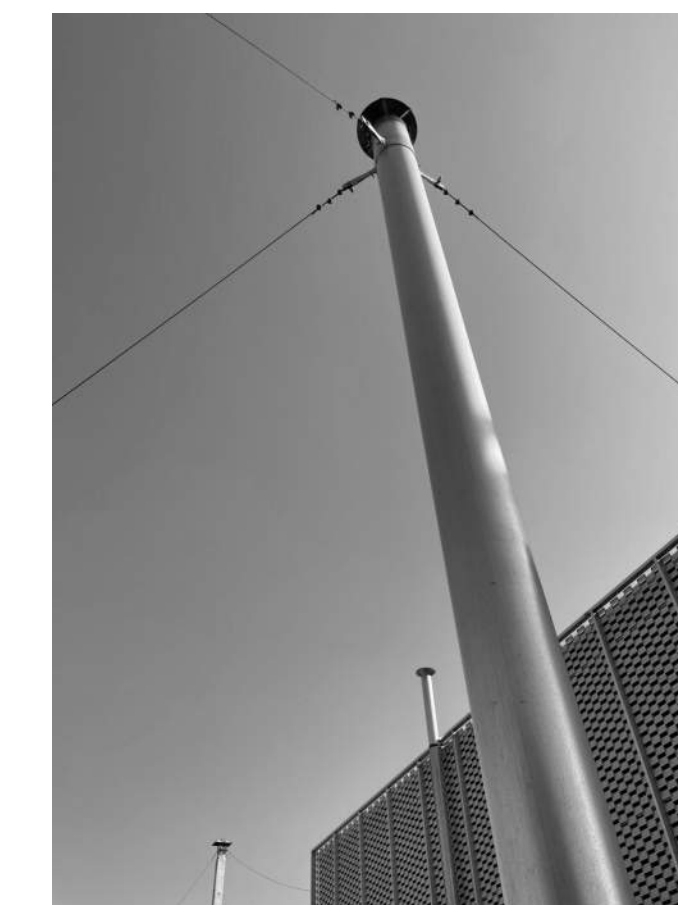
B.12 COORDINATE CHIMNEY TO REMAIN - CONFIRM NEW STAY CONNECTION POINTS. SEE NEW WORK KEYNOTE 15.
