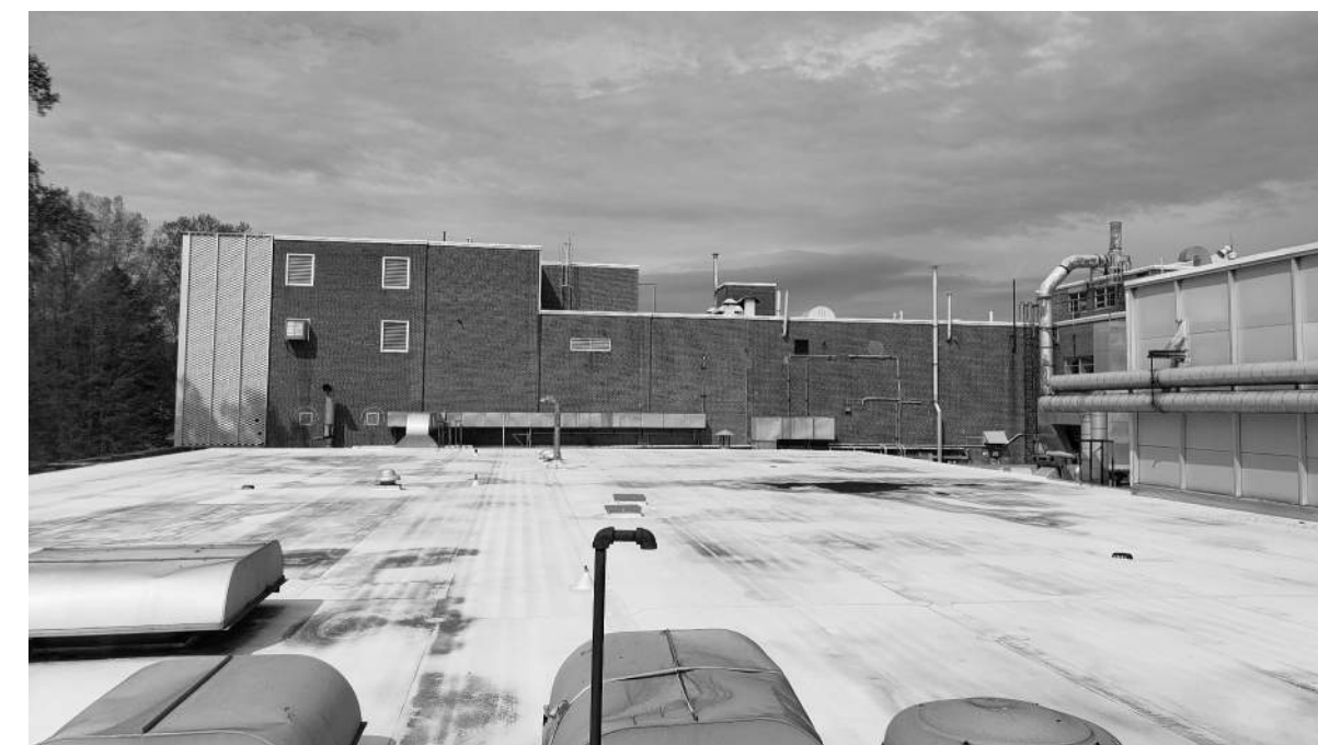
E.1 AREA E OVERALL FROM PLAN E. COORDINATE EQUIPMENT REMOVAL WITH PME DRAWINGS.
