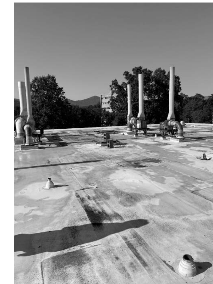
D.6 VIEW TOWARDS PLAN SOUTH. SEE PME DRAWINGS FOR EQUIPMENT TO BE REMOVED
