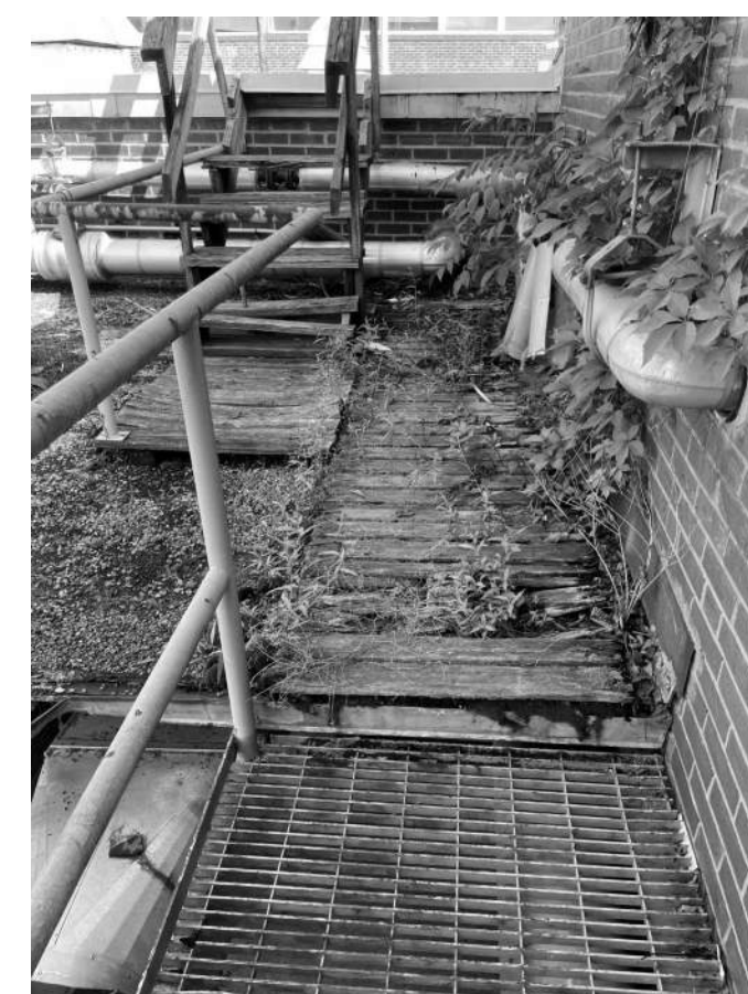
E.7 EXISTING CATWALK FROM CLASSROOM. TERMINATE GUARDRAIL AFTER FIRST 90°. STAIRS TO BE DEMOLISHED. NEW ROOF (COMPLETE TEAR OFF) ON AWNING.
