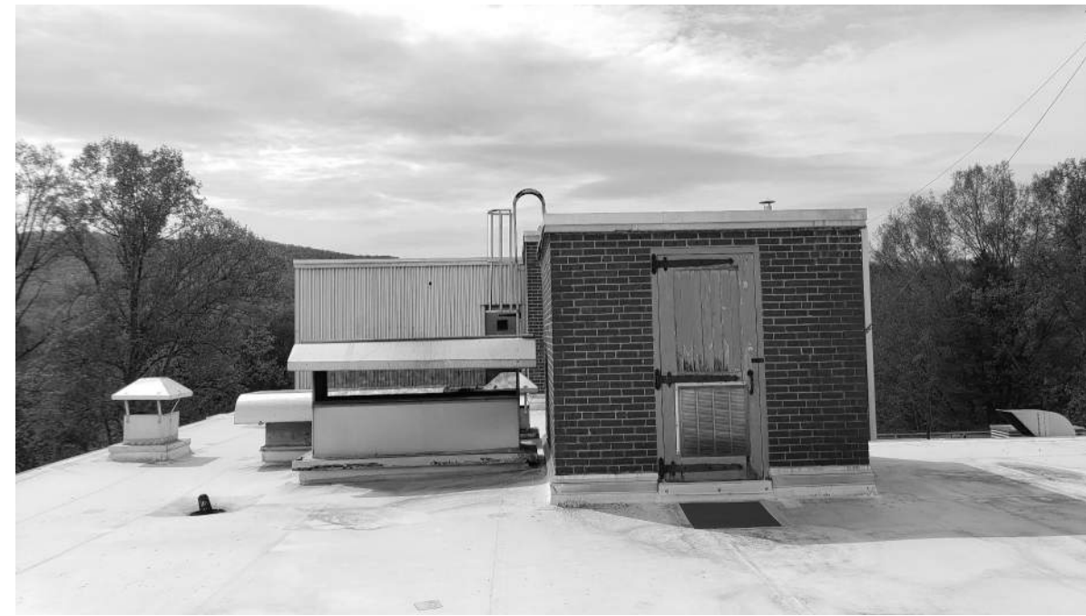
C.1 EXISTING PENTHOUSE TO REMAIN - REROOF IT AS WELL. COORDINATE EQUIPMENT REMOVAL WITH PME.
