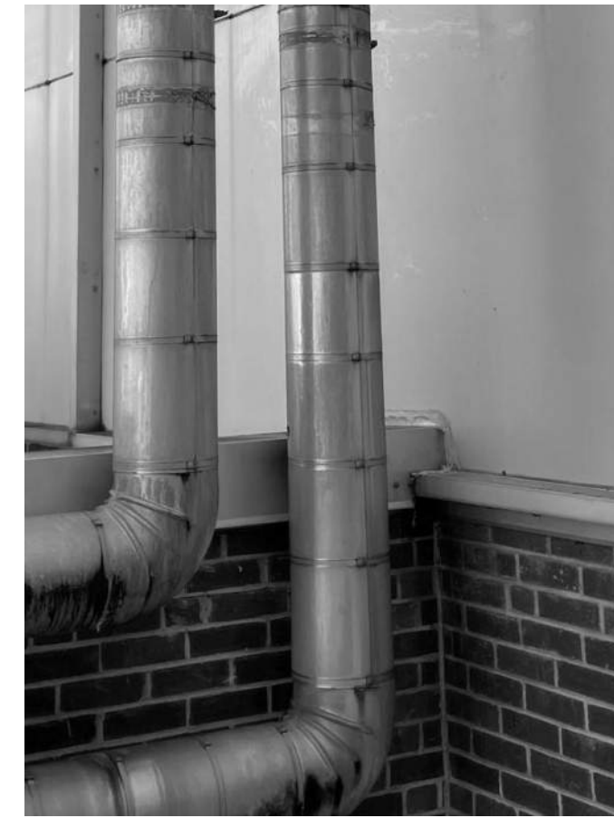
A.7 PIPING TO BE REMOVED. SEE PME DRAWINGS. NEW PARAPET CAP FLASHING AND END WALL FLASHING. SEE A4/A403
