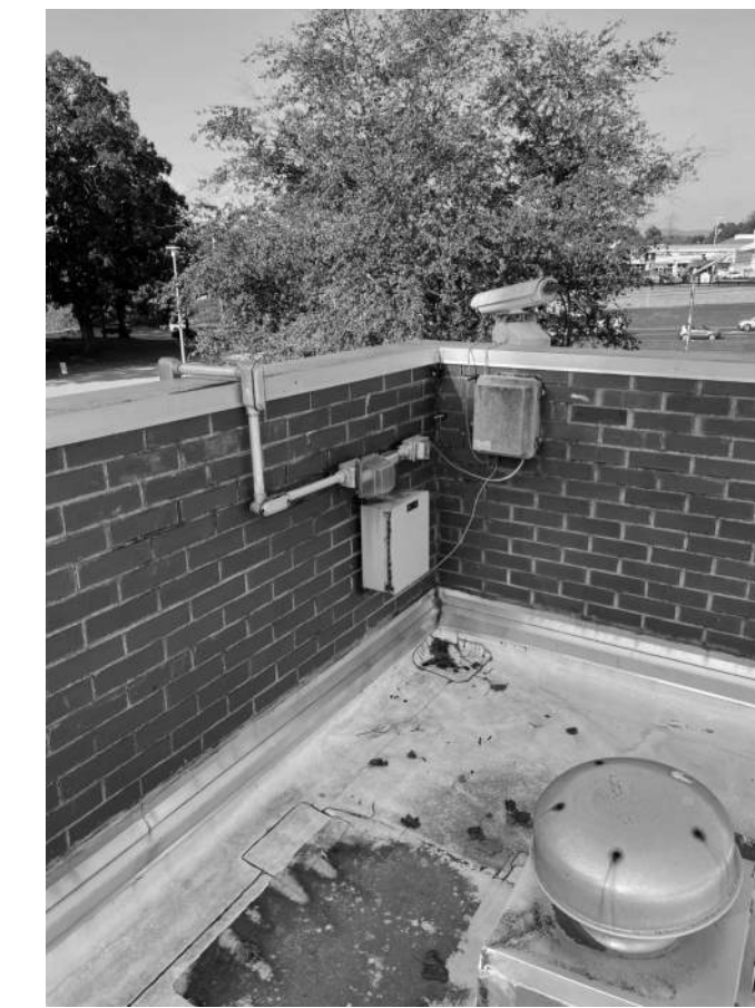
A.4 PARAPET TO BE REMOVED. COORDINATE EQUIPMENT TO BE REMOVED WITH PME DRAWINGS.
