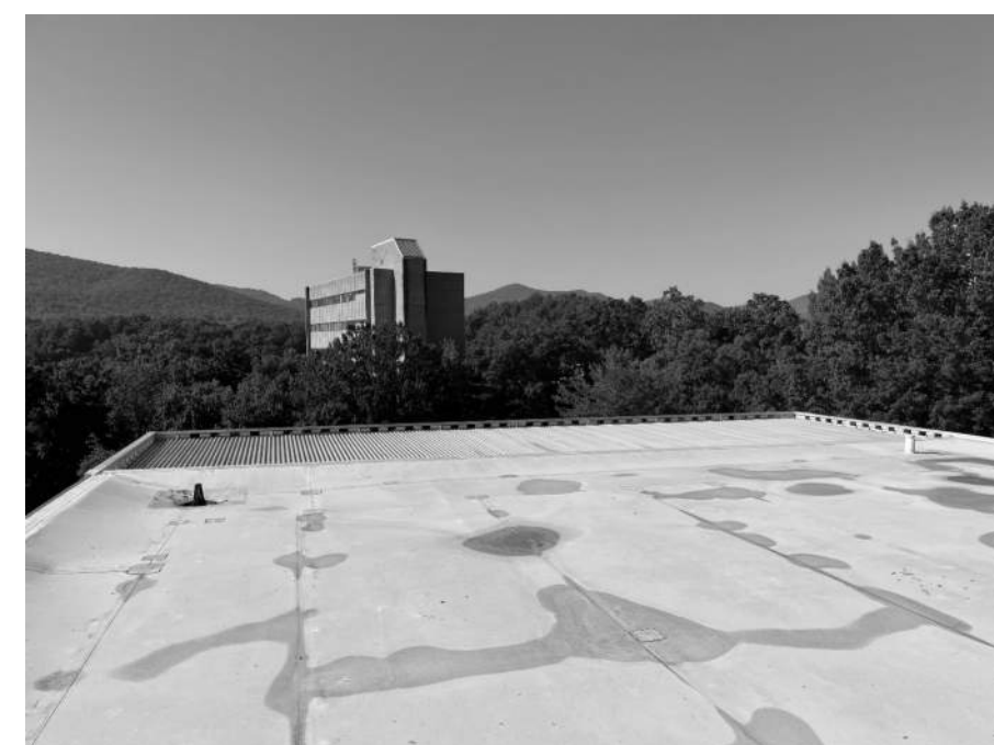
C.6 TOP PENTHOUSE ROOF. PLAN SOUTH. NICE VIEW. NO WORK ON METAL RIBBED ROOF.
