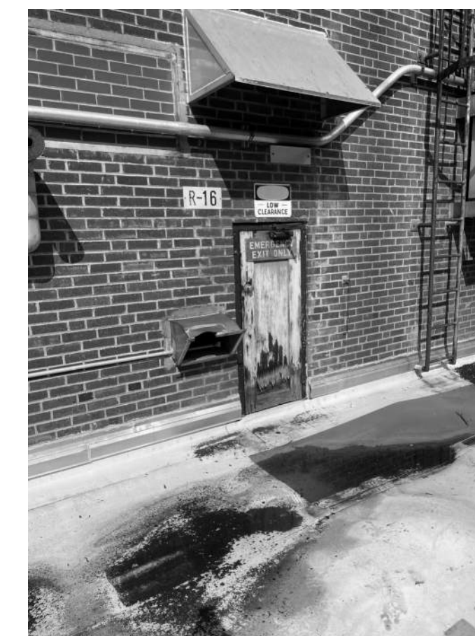
B.20 EXISTING DOOR AND FRAME TO BE REMOVED. REPLACE WITH NEW HM DOOR AND FRAME, MATCHING EXISTING HEAD HEIGHT, AND OVERALL WIDTH. SEE DOOR SCHEDULE ON A190.
