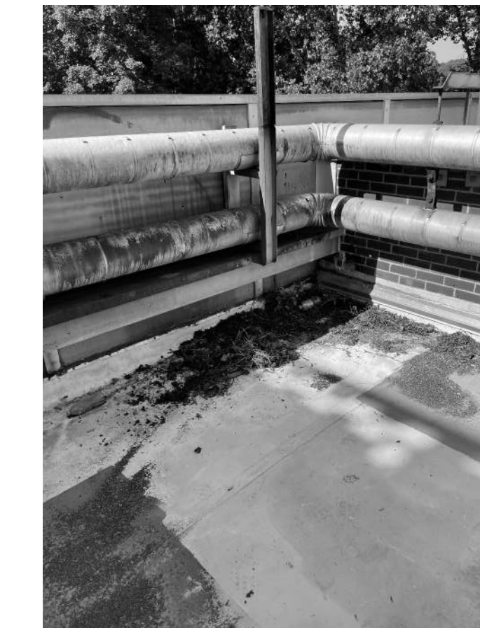
B.5 PIPING TO BE REMOVED. COORDINATE NEW FLASHING DETAILS. SUPPORTING STEEL TO REMAIN TO BE ENCOMPASSED IN TAPERED INSULATION
