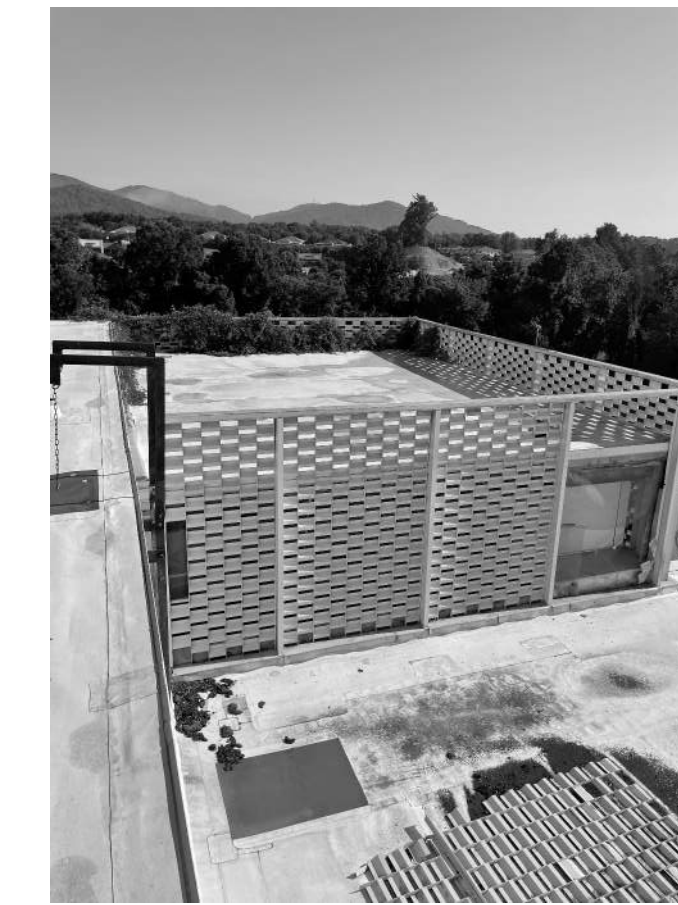
D.3 FLASHING TRANSITION AT PLAN WEST. SEE NEW DETAIL. PROVIDE NEW LADDER E6/A402
