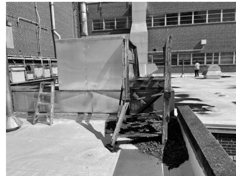
B.16 EXISTING STAIR TO BE DEMOLISHED. EXISTING DUCT ON ROOF TO HAVE NEW CURB. EXISTING DUCTING TO BE RAISED. SEE PME DRAWINGS.
