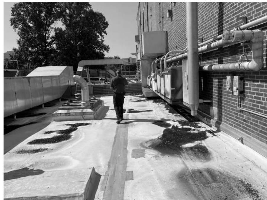
B.17 DUCTING ON RIGHT SIDE OF PHOTO TO BE RAISED ON NEW STANDS. SEE PME NOTES ON MAKING TRANSFORMERS (ON RIGHT) SAFE FOR WORK.
