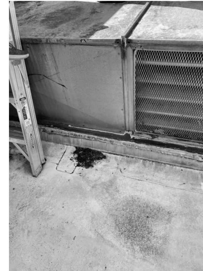
B.19 EXISTING DUCT TO BE REMOVED, ROOF MEMBRANE TO EXTEND UNDER, AND DUCTING REINSTALLED ON STANDS. SEE PME DRAWINGS.
