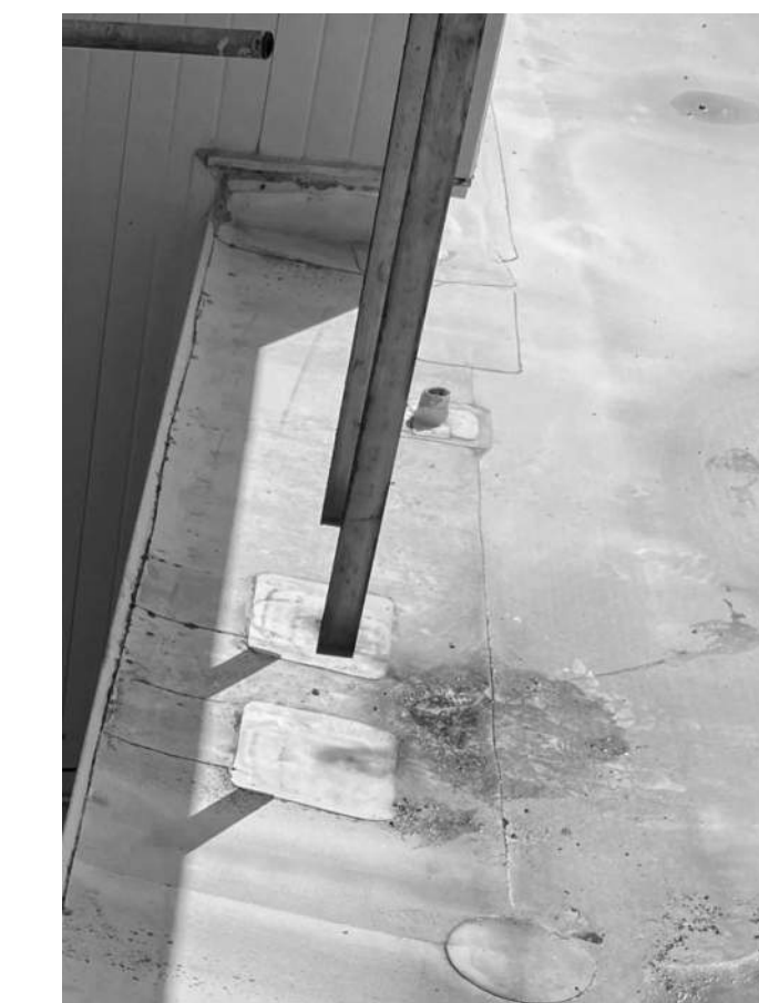
E.4 EXISTING FLASHING AT CORNER. SEE NEW FLASHING DETAIL C1/A402 (SIMILAR). LADDER TO BE REPLACED. SEE E6/A402.
