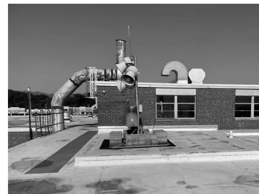
C.8 EXISTING LOUDSPEAKER SYSTEM TO REMAIN. COORDINATE WITH OWNER FOR TEMPORARY REMOVAL AND STORAGE DURING RE-ROOFING.
