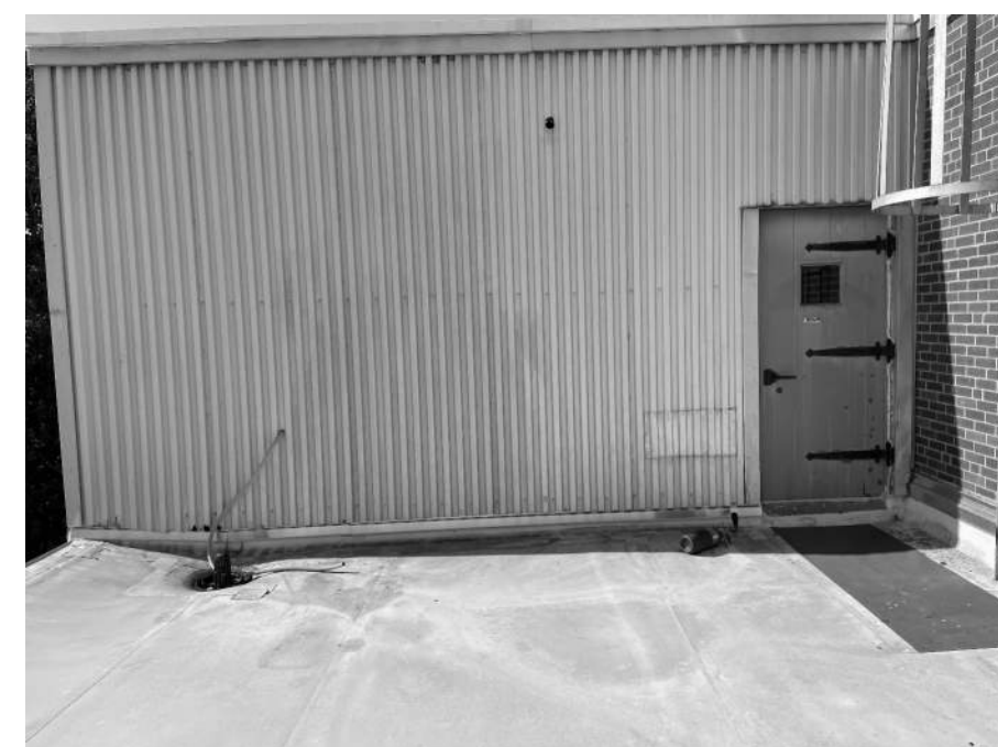
C.5 EXISTING METAL PANEL PER DETAIL A1/A403. TRIM DOOR AS REQ'D FOR NEW DOOR CURB DETAIL A1/A403
