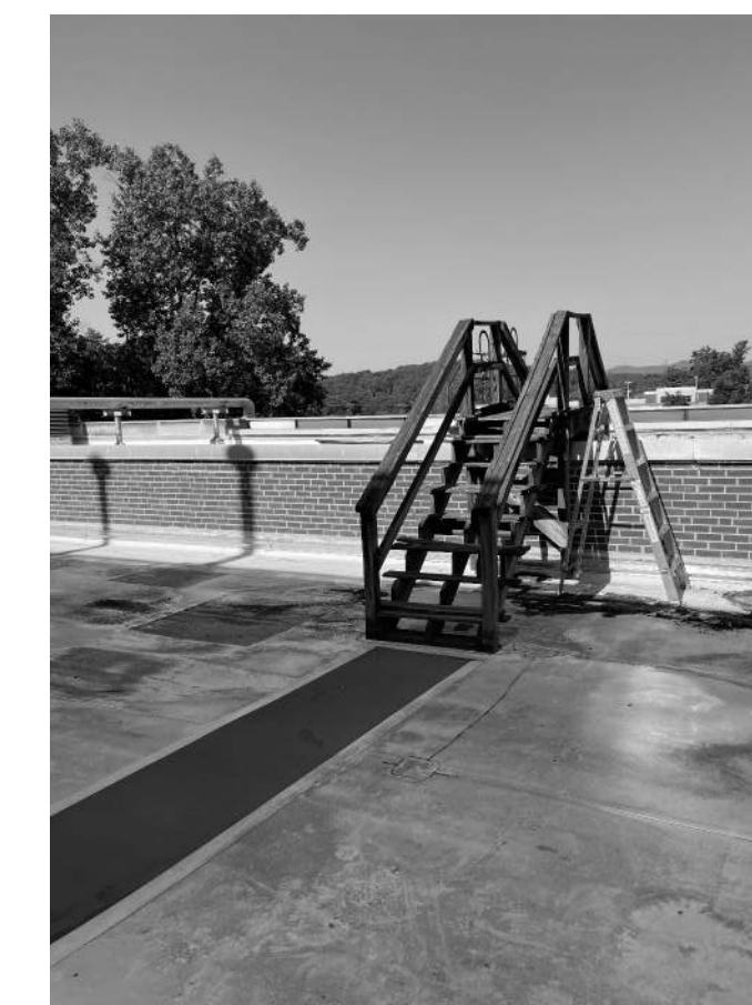
B.11 STAIR TO BE REMOVED AND REPLACED. SEE NEW STAIR DETAIL A9/A402.
