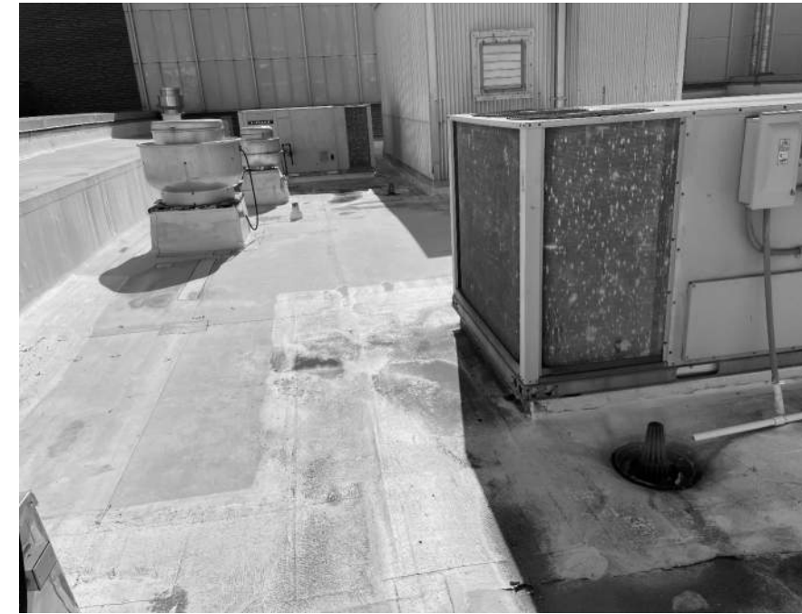
A.3 GENERAL VIEW - SEE PME AND ARCH FOR EQUIPMENT TO REMAIN. METAL CLAD PENTHOUSE BEYOND TO BE REMOVED AND DECK FILLED IN. SEE STRUCTURAL AND PME. NEW WORK KEYNOTE 7.
