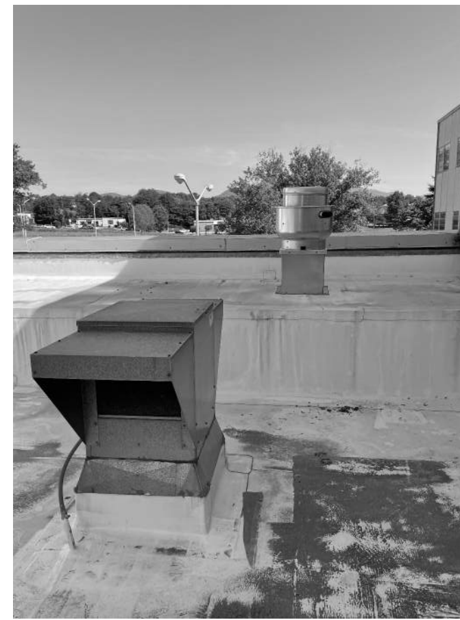
A2 DUCT TO BE REMOVED. EXHAUST THAT NEEDS NEW CURB. SEE DEMO KEYNOTE 6 AND NEW WORK KEYNOTE 5
