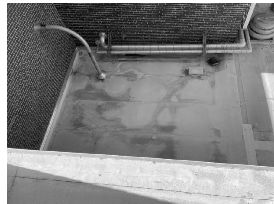
B.1 AREA TO BE SLOPED TOWARD MAIN DRAINAGE AREA. DRAIN TO BE ABANDONED.
